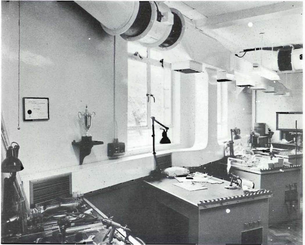
Photograph of Ducting System A
